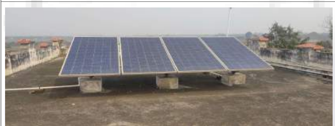
Solar Panel Installed at Rooftop
