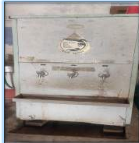
College Installed Water Purifier
