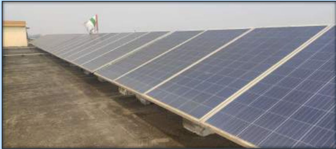
Solar Panel Installed at Rooftop
